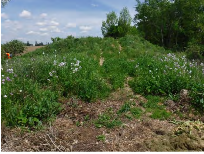
Plate 6: Berm of stripped topsoil piled at end of panhandle, facing northeast (Photo 7900)
