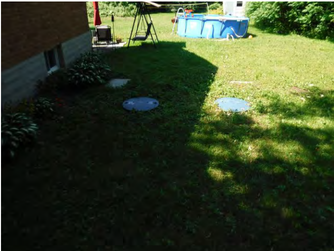
Plate 9: Lids of a buried septic tank northwest of the house, facing southwest (Photo 8052).
