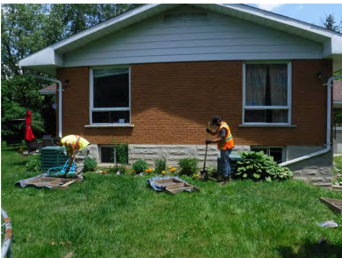
Plate 11: Shovel testing beside the south west wall of the house, facing northeast (Photo 8080).
