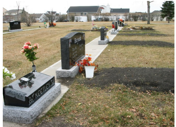
Concrete ribbon foundation for back-to-back casket lots without planting strip. (HLI design)
