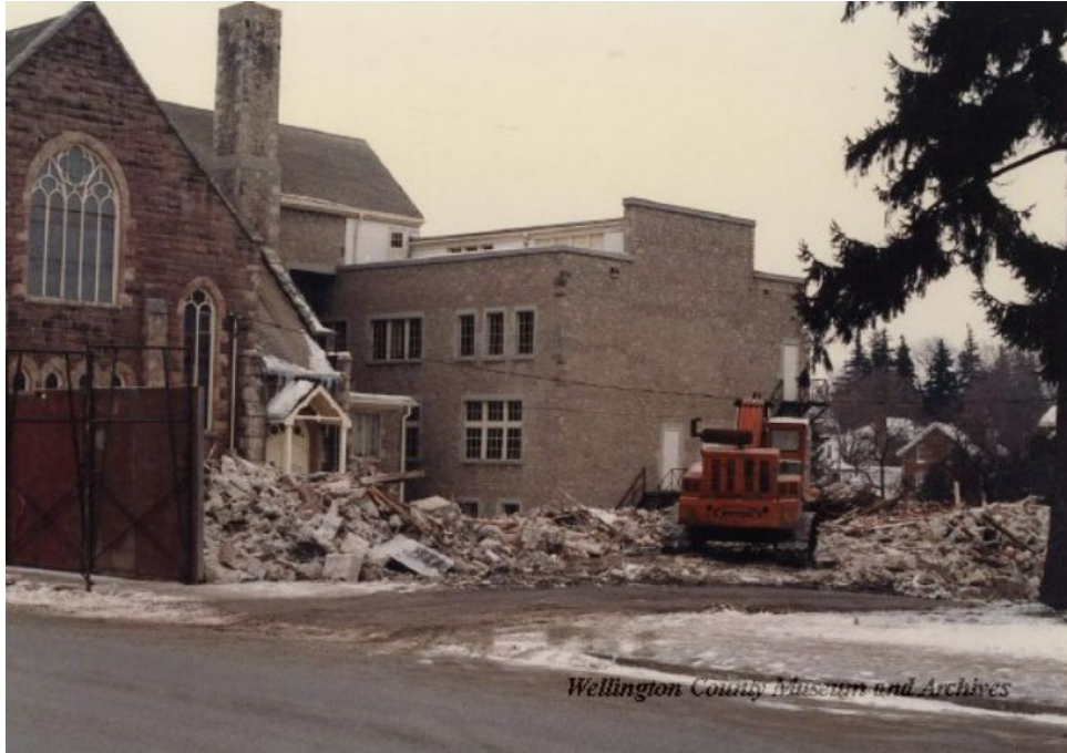
Figure 22: Rubble of the former Public Hall, demolished in 1983 (Source: Wellington County Archives & MHBC, 2022).
