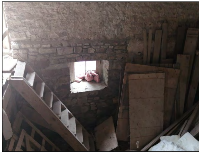
Figures 23 & 24- (above) View of progress of repair to masonry on west elevation; ((below) View of progress of repair on lower level of south elevation (Source: MHBC, 2022).
