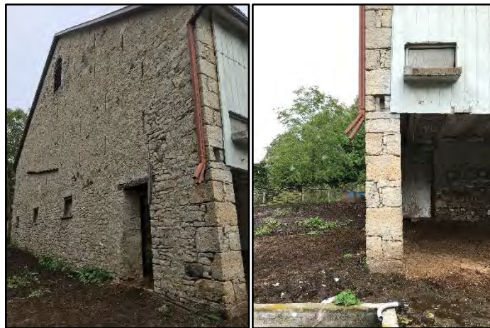
Figure 2: Mortar deterioration on exterior face of gable end wall
