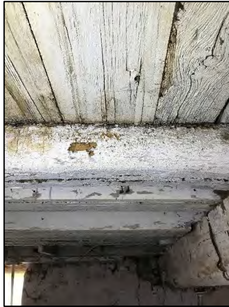
Figure 3: Joist deterioration in main floor framing
