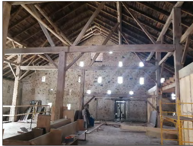
Figures 21 & 22- (above) View of the interior of the west elevation; (below) View of the interior of the east elevation also showing interior of wood roof structure (Source: MHBC, 2022).
