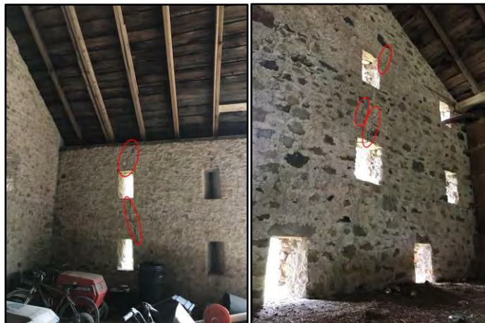
Figure 4: Cracking around openings on masonry walls
