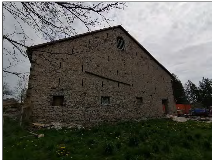
Figures 18-20- (left) The south elevation of the barn with gambrel barn addition (right) A view of the south elevation of main barn; (below centre) View of west elevation of main barn (Source: MHBC, 2022).
