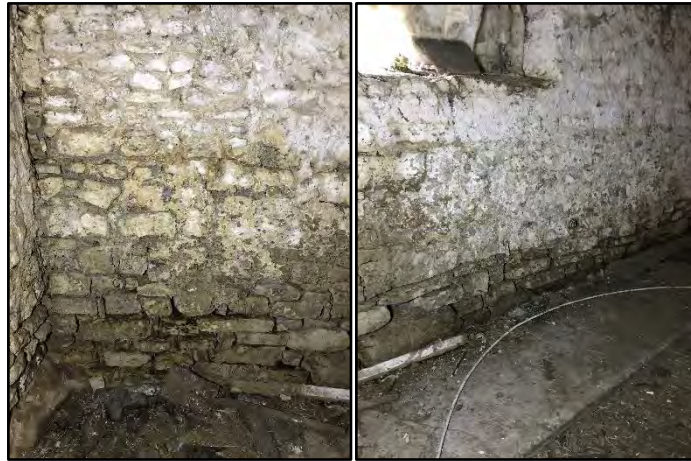
Figure 1a,b: Mortar deterioration of foundation walls
